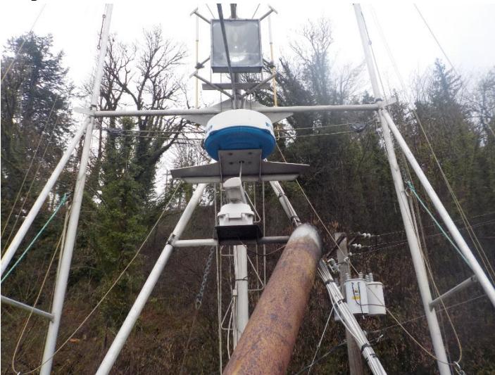
Figure 14 MAST AND LIGHTING
