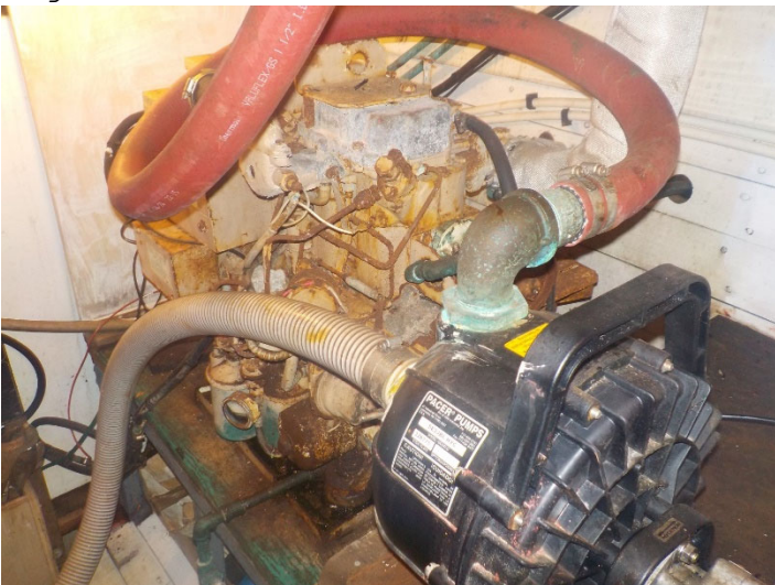
Figure 33 AUXILIARY ENGINE (NON-OPERATIONAL)
