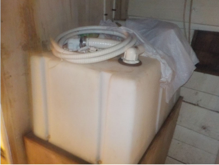
Figure 37 SEWAGE HOLDING TANK
