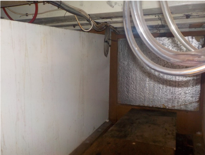
Figure 31 FUEL OIL TANK
